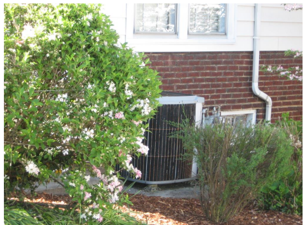
Appropriate screening of HVAC unit at 721 Yadkin Street.
