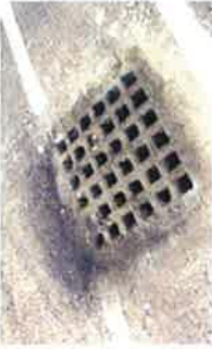
Grease evidence at storm gate. Grease was discharged into stream. Enforcement action was taken.
